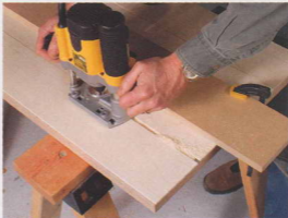
Rout the joint. To clean up any gaps, a router and edge guide are used to cut a shallow groove centered on the long joint.
